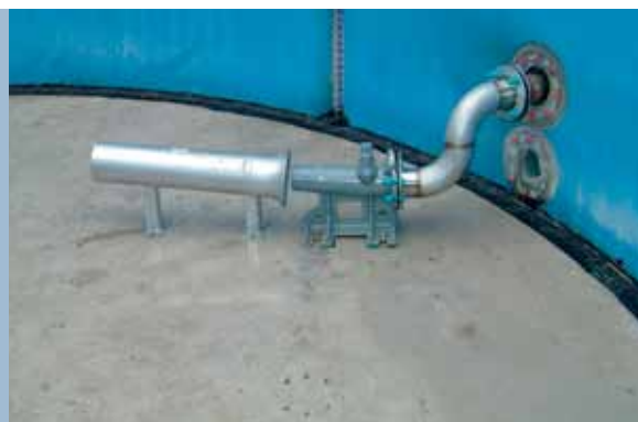
Inside the tank: The nozzle and ejector pipe are located to generate a bulk flow loop, which leads to re-suspension and homogenization of the mixed sludge.
